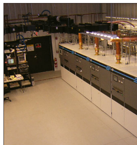
The Acrodyne Quantum transmitter at the WWAZ-TV site in an example of a clean, clutter-free installation.
