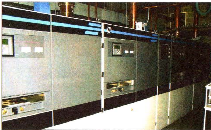
WBUW installed a four-cabined Acrodyne/Ai Quantum transmitter, the biggest that the company had built up to that point.
